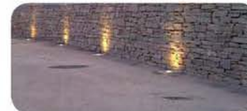
Wall wash luminaires
