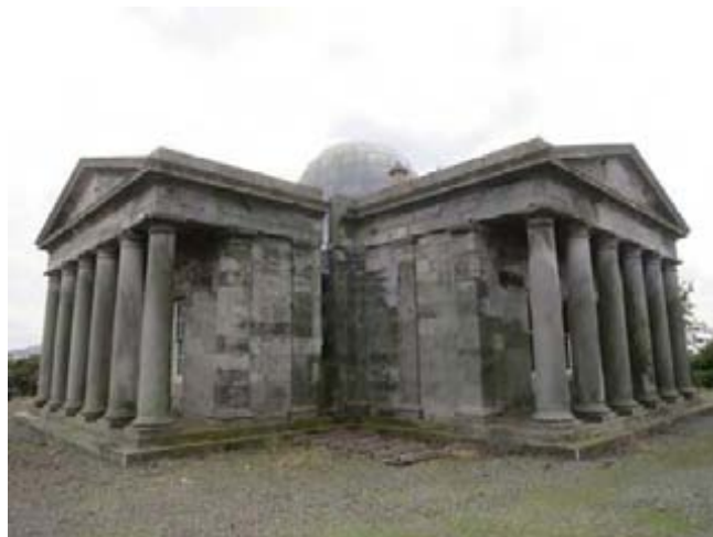
North east corner indicating vegetation growth on stonework
