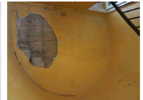
Ceiling damage over stair
