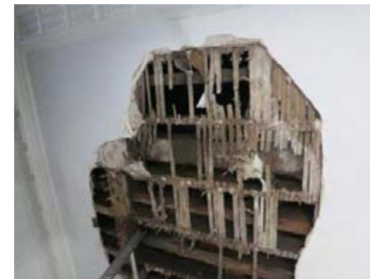
Ceiling damage in central hall
