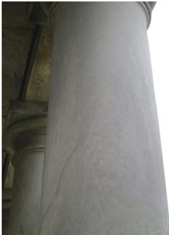
Stone column with diagonal fissure
