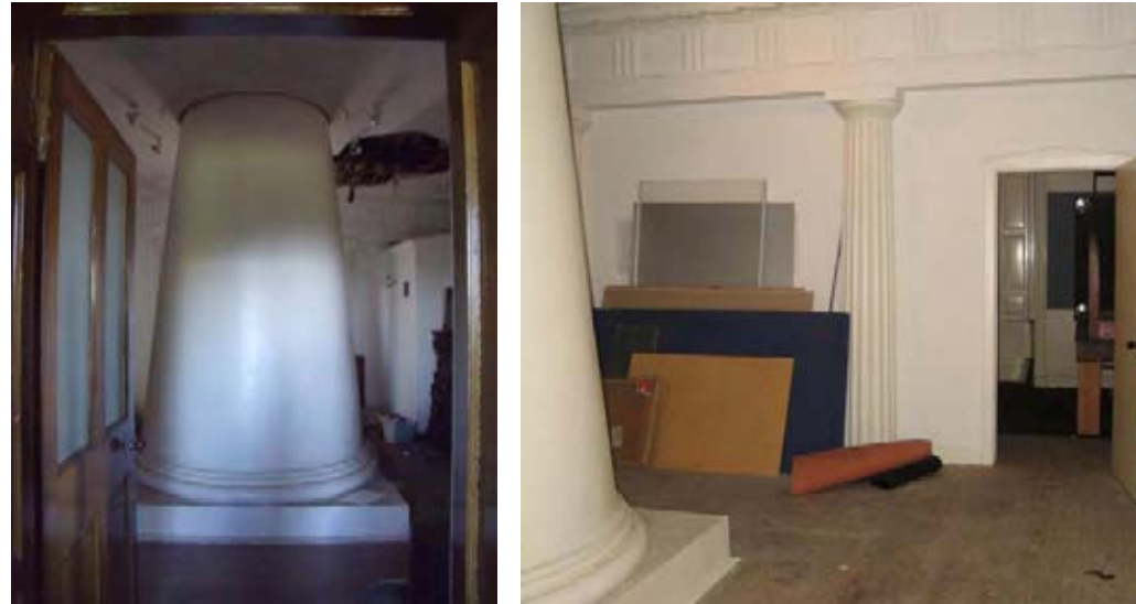
Central Hall, currently overly dominated by central column, supporting telescope above, due to addition of partitions subdividing space and removal and adjustment of columns now offset with cornice above.
