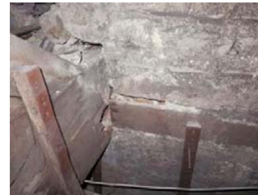
Rot at truss bearing
