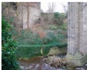
Retaining wall under Dean bridge. Most of the riverbanks have retaining structures along them, not benefiting from design by Telford but similarly affected by ivy
