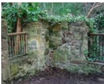
Cracked walls, ivy, rotten handrails and rusty railings at Lindsay's mill space
