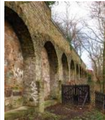
Retaining wall at top of India Street bank and below Doune Terrace Gardens
