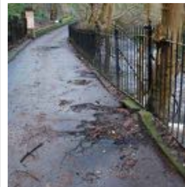
Walkway surface and retaining wall damaged by tree roots
