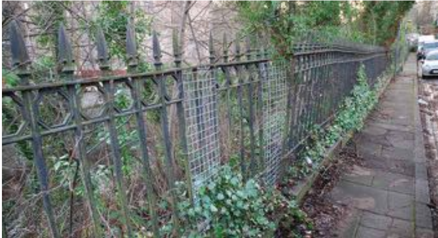
Railings and copes in very poor condition, Dean Terrace
