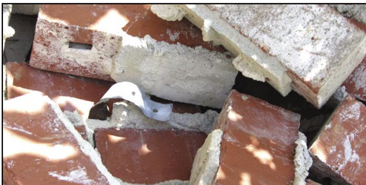
Figure 3. This tie remained embedded in the mortar joint while the smooth-shank nail pulled from the stud.
