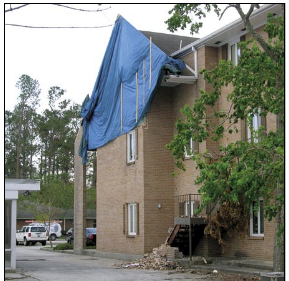
Figure 2. The upper portion of the brick veneer at this apartment building collapsed. Pedestrian and vehicular traffic in the vicinity of the damaged wall were vulnerable to injury and damage if remaining portions of the wall were to collapse during subsequent storms.
