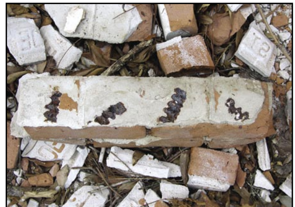
Figure 6. There were several ties in this portion of the wall, but they failed due to severe corrosion.
