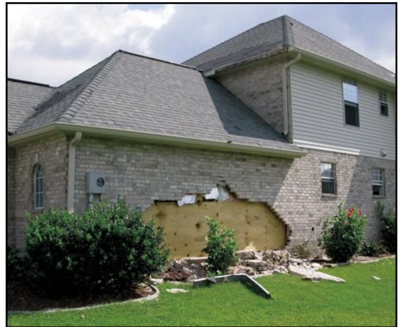
Figure 1. Failed brick veneer. Plastic foam wall sheathing was installed over the wood studs (plywood was temporarily installed after the brick failure).
