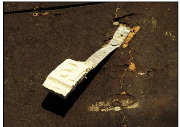
Figure 5. This tie was embedded in the mortar, but the bond was poor.
