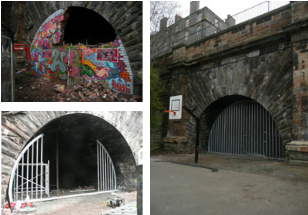
FIG 21 Demolition of brick infill (used for organised graffiti artwork activity with local children prior to demolition) and installation of new metal security screen.
