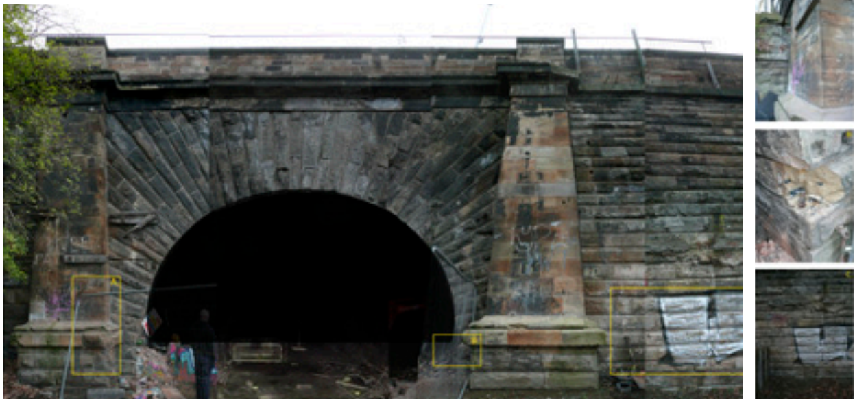
FIG 23 Initial identification of stones requiring repair or replacement with close-ups right. The photo was taken following demolition of the brick infill and prior to the installation of the metal security screen.
